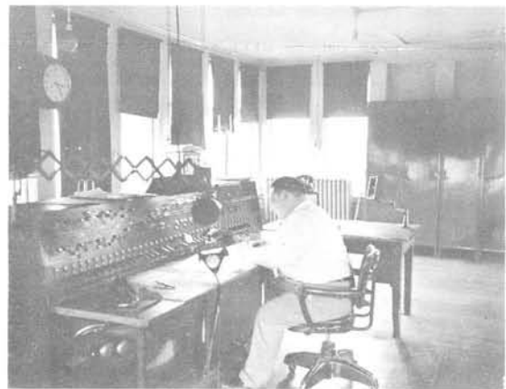
Dispatcher Don Robinson working the second trick at the Boston and Maine's "DI" tower at Gardner, Mass. C.T.C. board controls main line from Athol to South Ashburnham on the Fitchburg Division.
