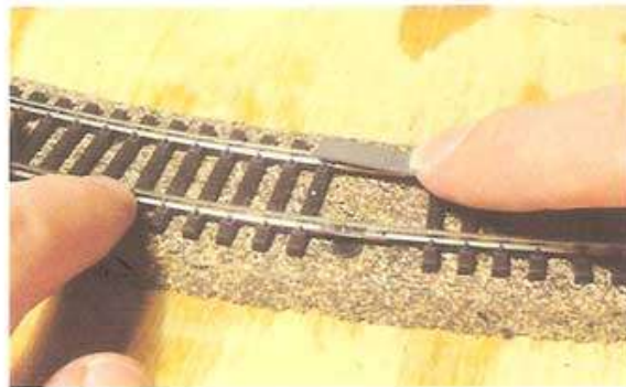
Fig. 9-20. Give the railhead a couple of passes with a needle file to make sure the joint is smooth.
