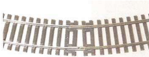
Track joint forced into a too tight radius. Note open joint.
