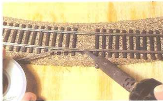
Fig. 9-18. Make sure the joint is tight and square, then solder the rails at each joint.
